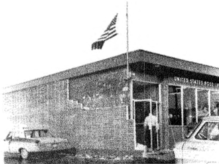
Figure 12-1 Damaged brick veneer can be a falling hazard. Post Restricted Use and barricade unsafe area.
