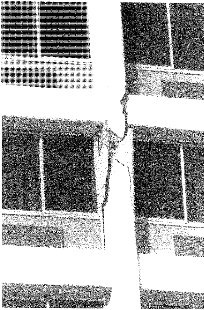
Figure E-17 Close-up of fractured column from Example 4. This column, which lacks confinement of the vertical reinforcement, has essentially lost its capacity to carry a vertical load.
