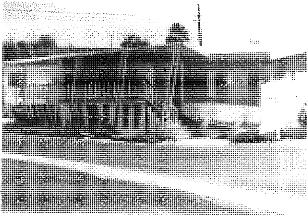
Figure 10-2 Mobile homes that are not braced between the foundation and the undercarriage often collapse in strong shaking. Damage to this mobile home not only includes collapse of vertical supports, but also damage to the undercarriage and porch. Post Unsafe.
