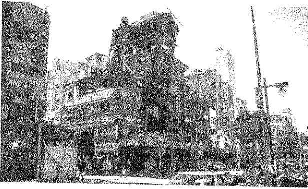
Figure D-3 This office building in Kobe, Japan, is considered an unstable Unsafe structure because it could easily collapse in an after-shock. Entry is not allowed.
