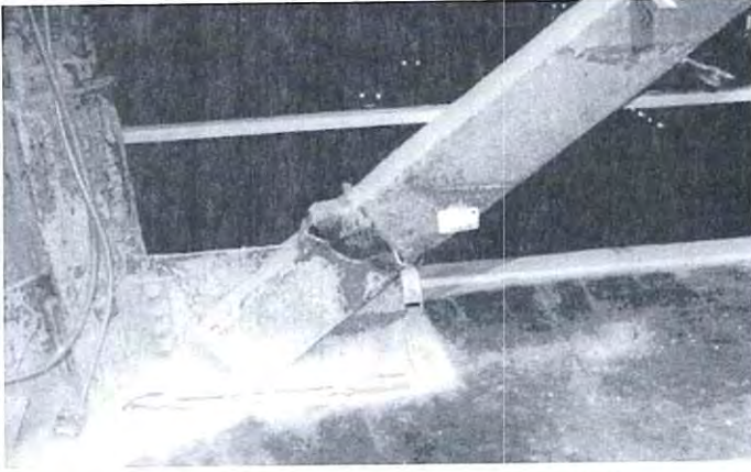
Figure 9-7 This steel tube brace has completely failed. There were few signs of distress until the wallboard finish and fireproofing were removed.
