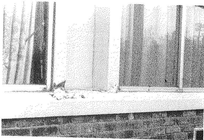
Figure E-5 Spalling at mullion, Example 2.
