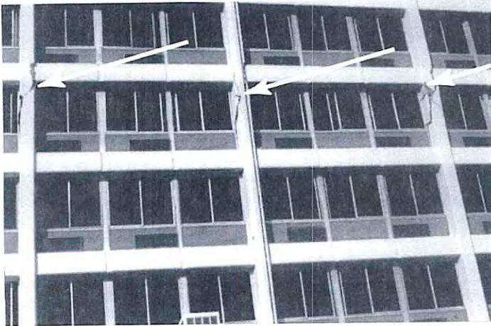
Figure E-16 Columns between the fourth and fifth floors are fractured, Example 4.
