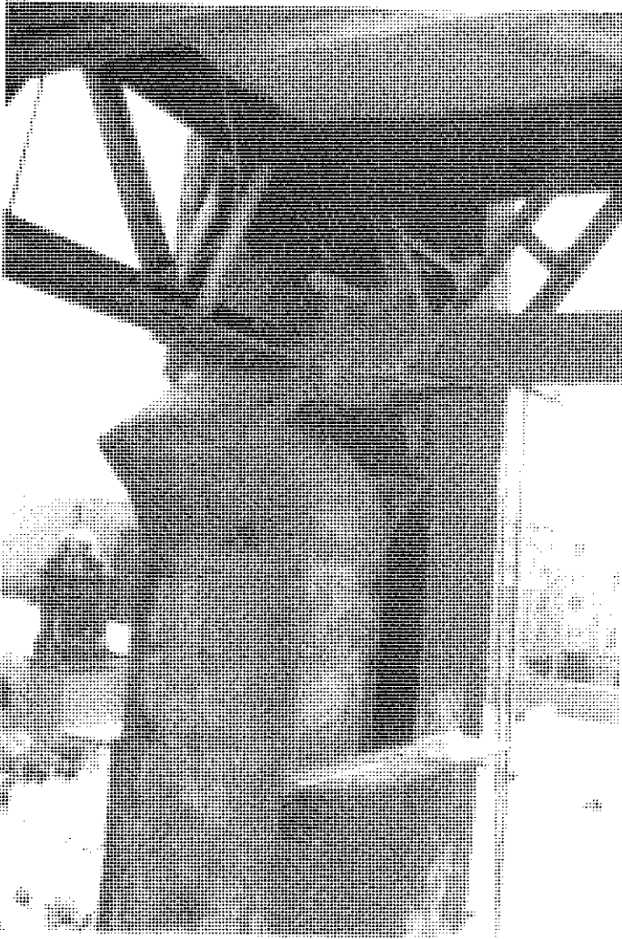
Figure 9-4 Local column buckling of this type constitutes a clearly unsafe situation. Post Unsafe.
