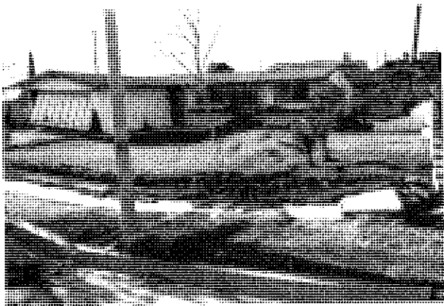
Figure 11-3 House damaged by ground displacement caused by surface faulting from the 1971 San Fernando, California, earthquake. Post Unsafe.
