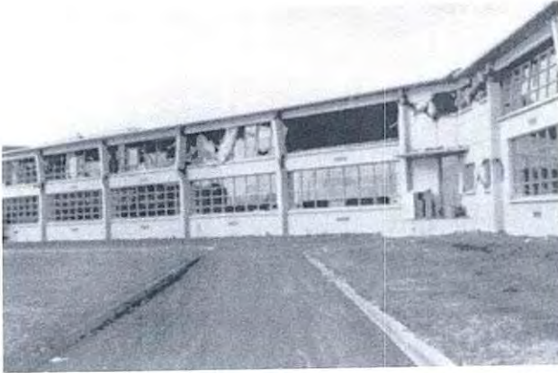
Figure 8-7 Failure of concrete columns with top and bottom hinging. Post Unsafe.
