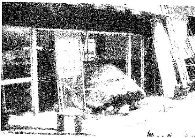
Figure 11-5 Damage to store front caused by rock fall.
